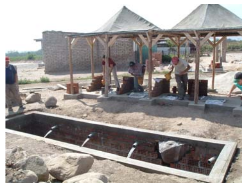
Demonstrating the flushing of the toilets during building and disposal system construction.
