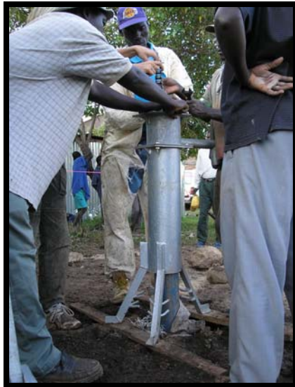
Figure 7 - Installation of the India Mark II hand-pump
