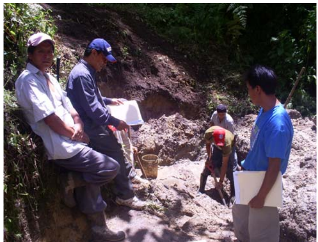
PAVA staff member René Martínez collaborates with local and municipal workers studying pipeline placement.
