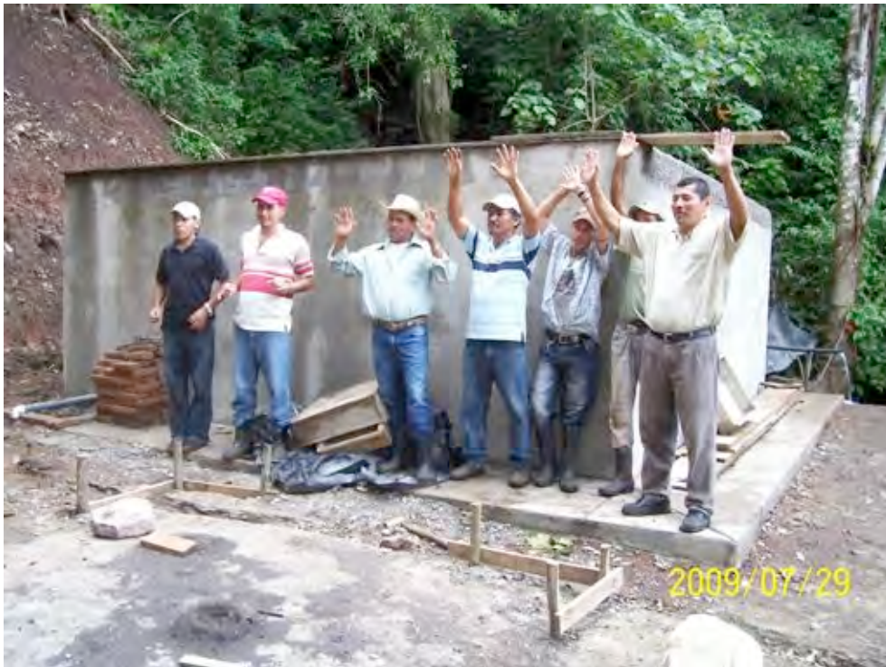
Figure 1: New distribution tank (lower) and several Community Members in Payacuca
