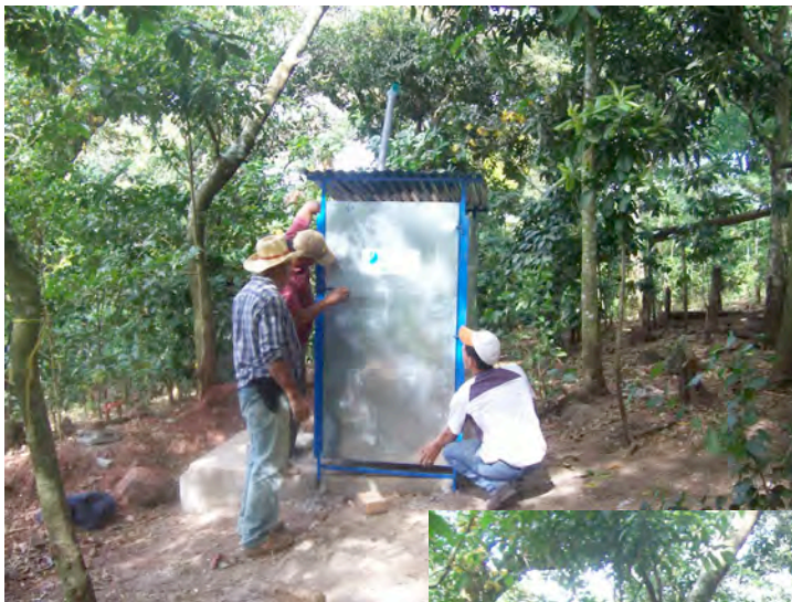
Phase 2 latrines in Payacuca: The concrete that extends to the left is the second pit of the double pit latrine.
